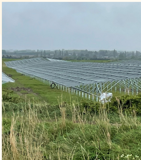
The support structures for the solar panels following the contours of the landscape
